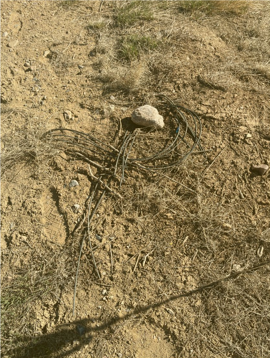
Photo 9: Evidence of irrigation in disrepair
