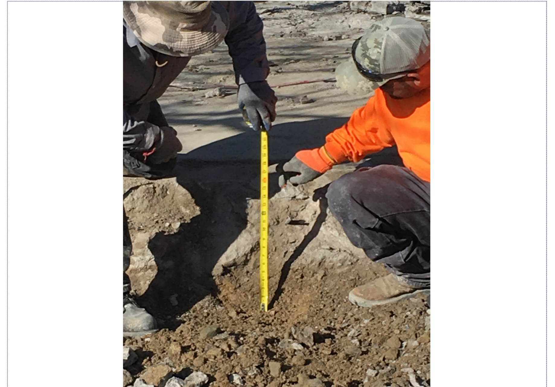
Concrete thickness over 10". Fill dirt and road base were added to allow for 6" of concrete to be poured per the scope.
